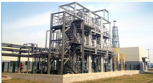
Waste stripper and waste solvents recycle system
