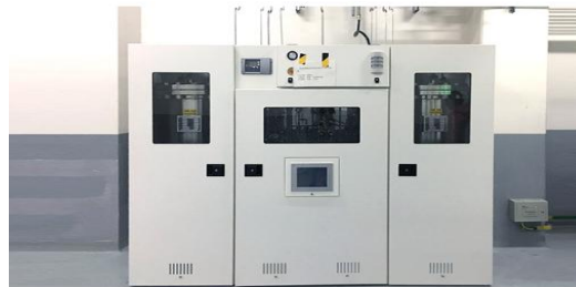
Special gas supply system
