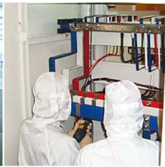
Electromechanical and Air-Conditioning Engineering
